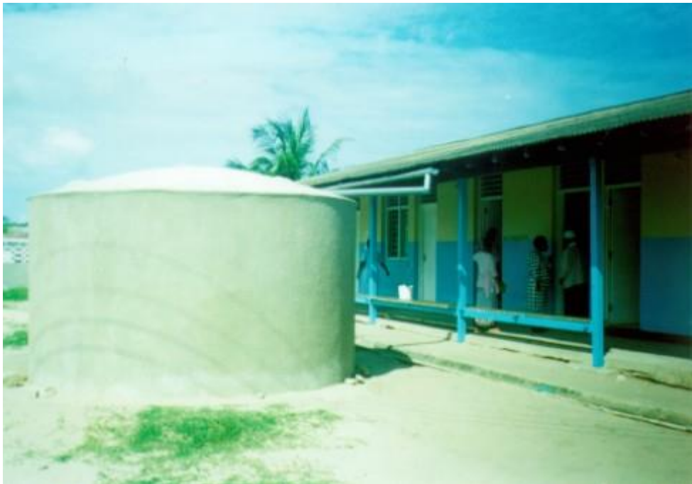
Figure 3: Demonstration rooftop catchment system at Mburahati dispensary, Dar es Salaam
