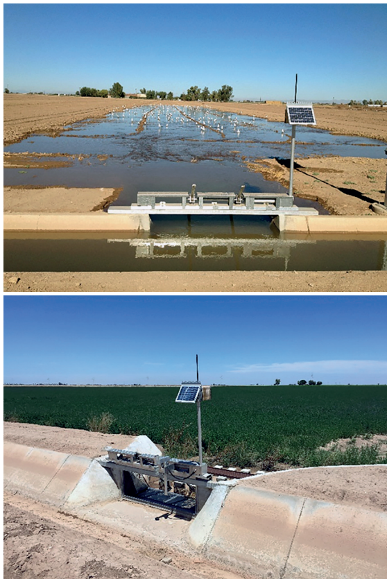
Figure 2. Surface irrigation automated gates in Holtville, California.
